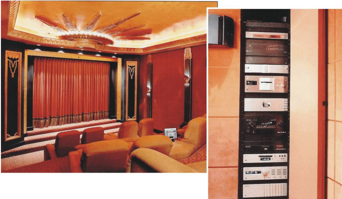
Figure 1 – A $600,000 home theater, with Stewart 150" FireHawk screen, Sony Qualia 004 SXR projector, Sony 400 DVD Changer with ReQuest management, Lexicon Audio, Revel Ultima Speakers, and Crestron automated controls for Audio-Video, lighting, shades and heating. A CEDIA Electronic Lifestyles award entry.
